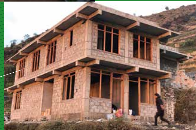
Continued construction of new two-story health center in Hagam, Nepal (due to open in 2022)
